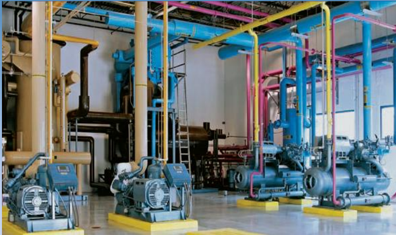
Site-Built CO 2 Cascade Refrigeration Systems
